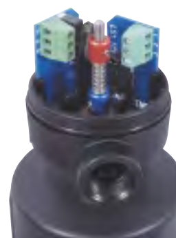
Internal View of Limit Switch Box
